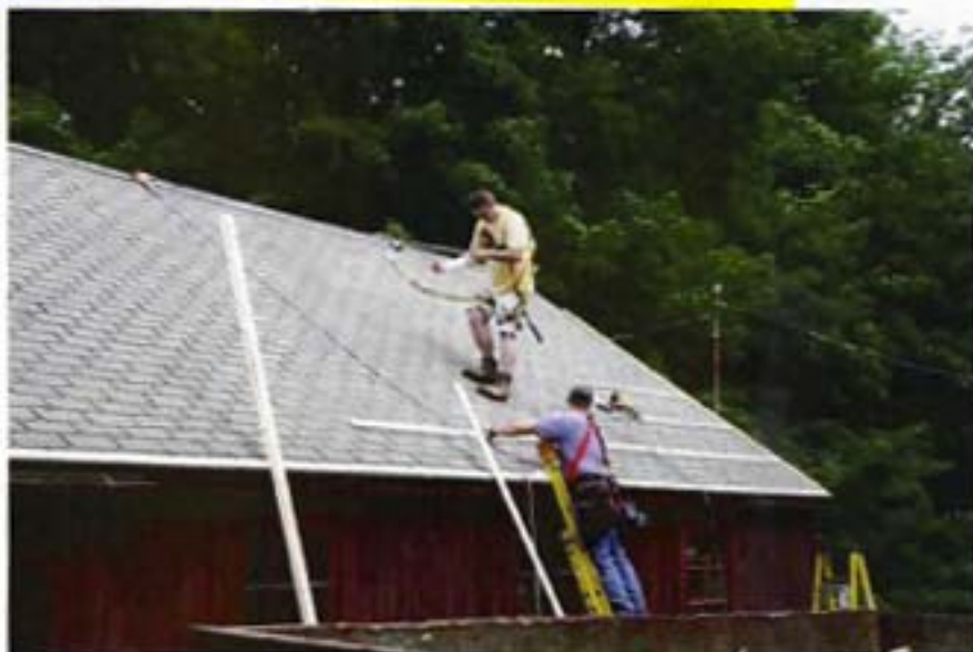
Ted Dickinson (roof) and Mike White (ladder) of Cobb Hill Construction, Inc. take safety precautions while strapping an old garage/barn roof in preparation for a new metal roof in Hopkinton, NH.
