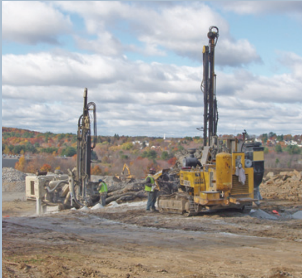
Maine Drilling and Blasting uses Atlas Copco ROC 748 and Ingersoll Rand 590 drills on J. Masterson Construction Corporation's Haverhill Commons job site.
