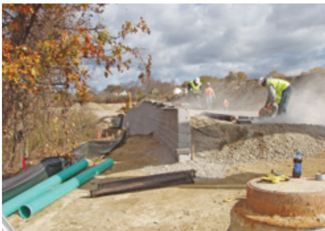
One of six Versa-Lok retaining walls is erected. Walls total 28,000 square feet.
