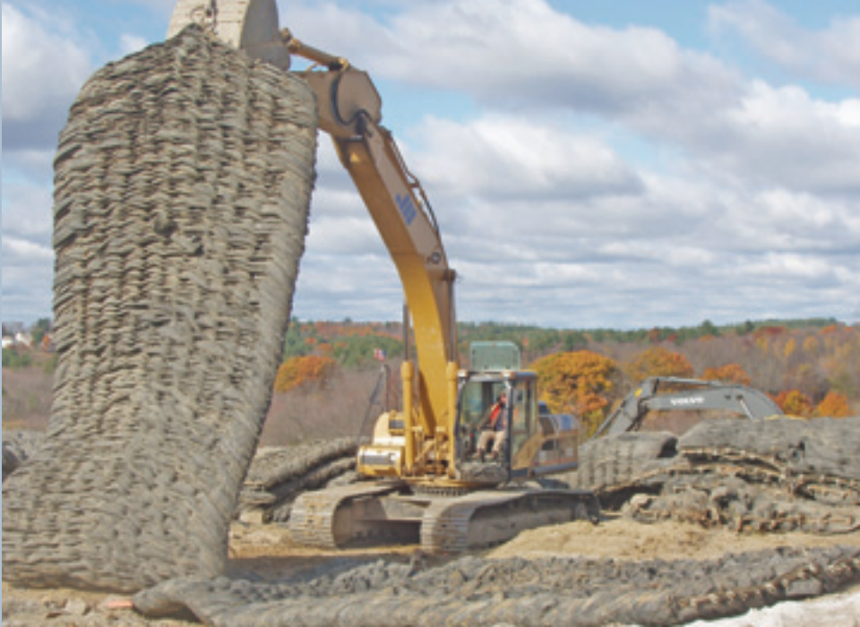
Left: CAT 330C excavator moves a blasting mat to cover the next shot.
