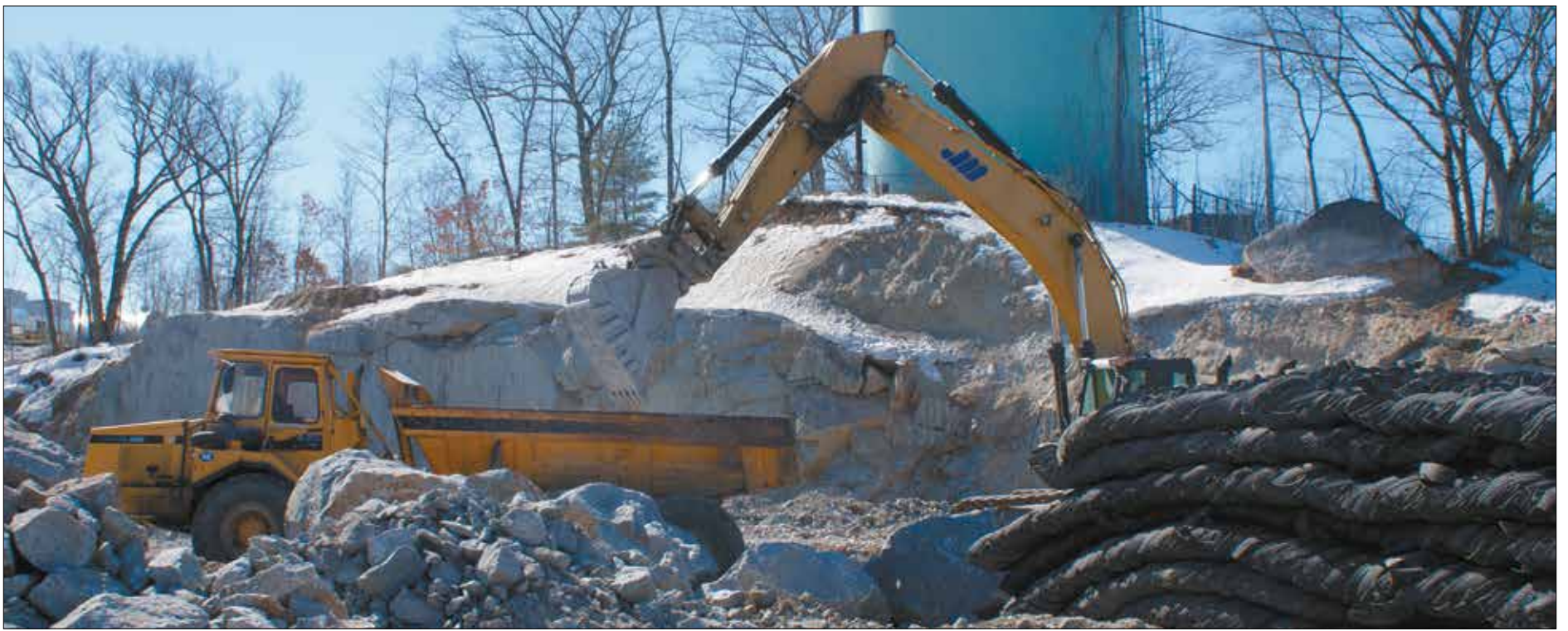
Excavator loads rock blasted out near municipal water tower onto a Volvo BM off-highway truck.
