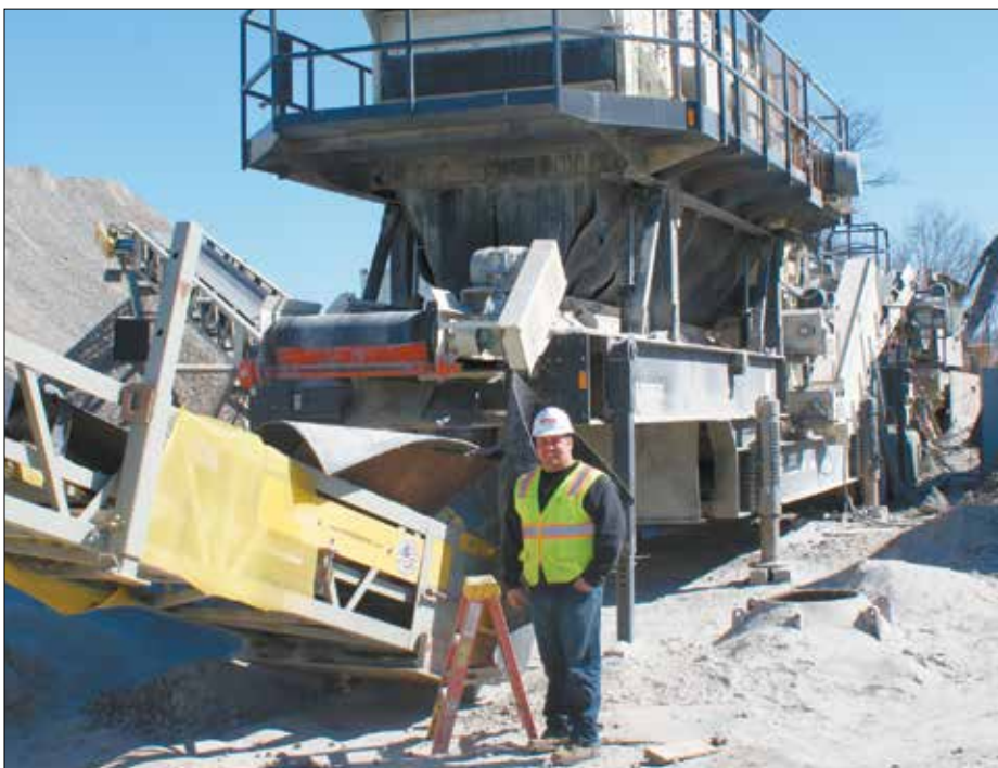
CM&B Assistant Project Manager Derek Harmon is flanked by TEREX/Cedar Rapids GRC380HLS rock crusher used to process blasted rock.
